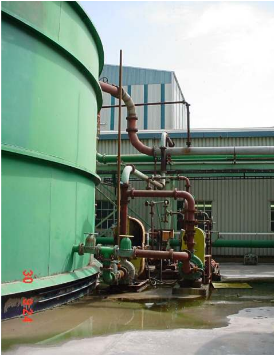
Centrifugal pump with stand pipe fitted
